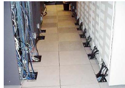
Seal cable cutouts
